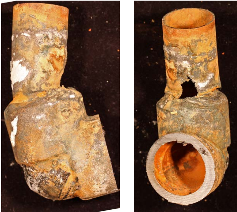
Figure 5. Additional views of elbow and leak after sectioning from line
