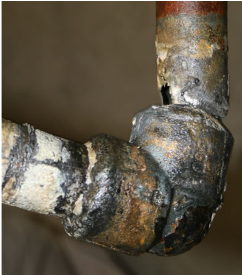
Figure 4. Leak site after removing fiberglass patch
