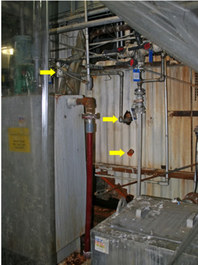
Figure 1. Sulfuric acid tank and piping
