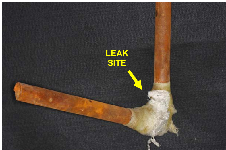
Figure 3. Location of leak in failed section of piping, as-repaired in field
